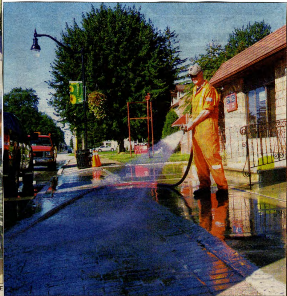
WASH OUT JEFF KEMPENAAR/CHRONICLE Jack Fisher from the West Elgin road department washes cement dust from the bricked sidewalk in front of the Canada Post office on Main Street in West Lorne Monday. Residents have been complaining about sidewalk dust, weeds and a poorly maintained streets.
